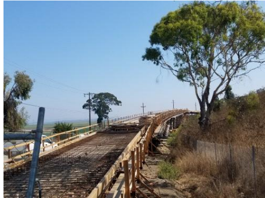
He also worked on the Castroville Bicycle and Pedestrian Overpass Project in North Monterey County.
